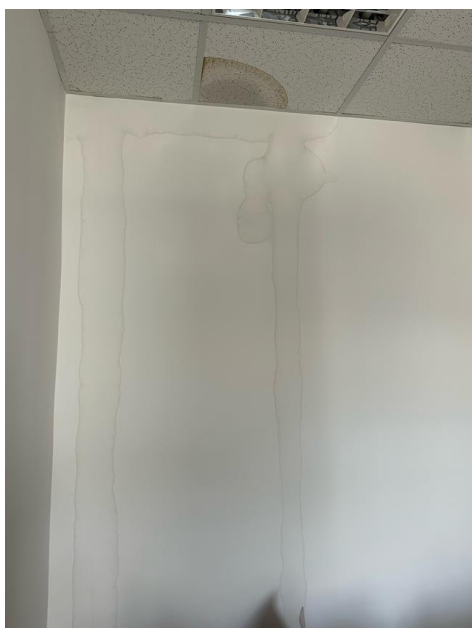
Figure 7. The observed leakage on the wall
