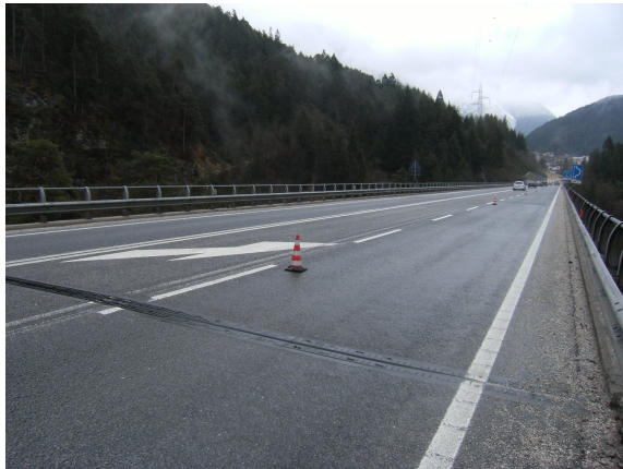
Figure 5: Road bridge located in Perarolo di Cadore considered in as test case in this work.
