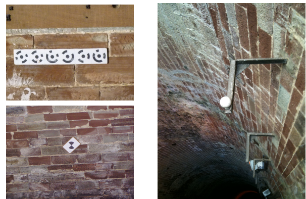
Figure 4: Encoded target for the photogrammetric model (top-left) ; black and white target (bottom-left) ; sphere (right). Encoded targets and spheres are located on the right side wall and black and white targets are fixed on the left side wall.
