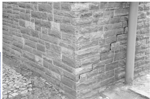
Figure 12. Regular photography showing structural damages on the wall
