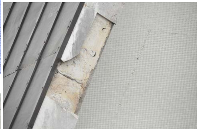
Figure 13. Regular photography from structural damages and missing or broken marble plaques
