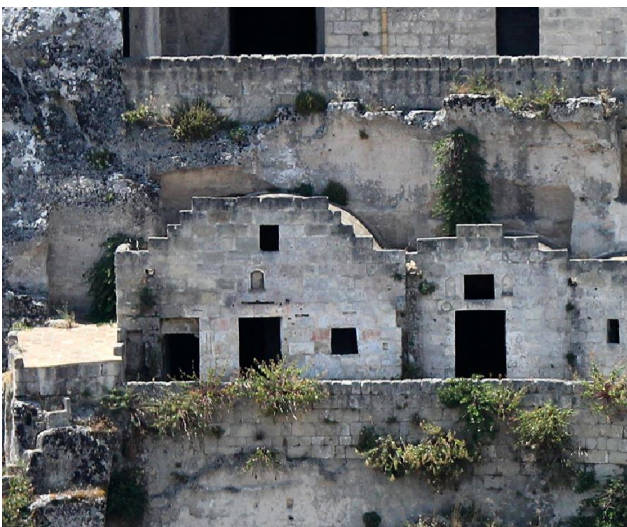
Figure 13. The elevation and the absence of the closures
