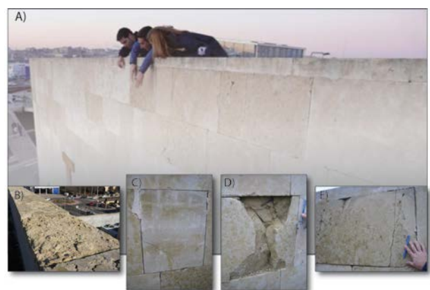
Figure 1. Villamayor Stone decay. A.- Southwest cladding façade with significant decay of the Villamayor Stone. B.- Material loss and scaling in the copings of the cornices. C.- Fissures in the grained Villamayor Stone. D.- Fissures and material loss in the clay-fine Villamayor Stone and its anchoring. E.- Fissures and cracking in the clay-fine Villamayor Stone below the coping of the cornice.
