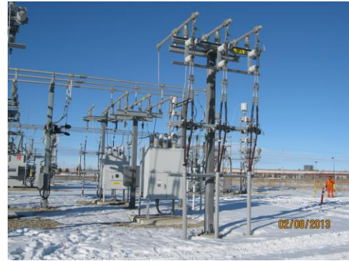
Figure 2. The scanned electrical substation in Airdrie
