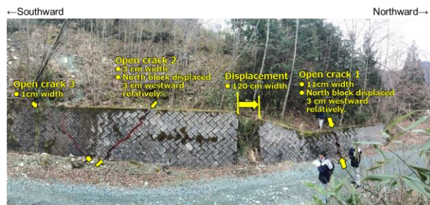
Figure 7. Field photo in Motoyama-b site. Concrete block wall beside a forest road had some open crack and displacement.
