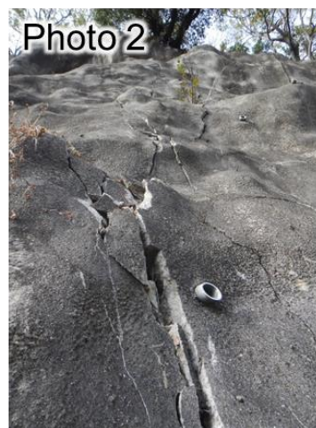
Figure 5. Field photos in Tanabe site. (Photo 1: road replacement, Photo 2: fresh open crack of mortar spraying wall)
