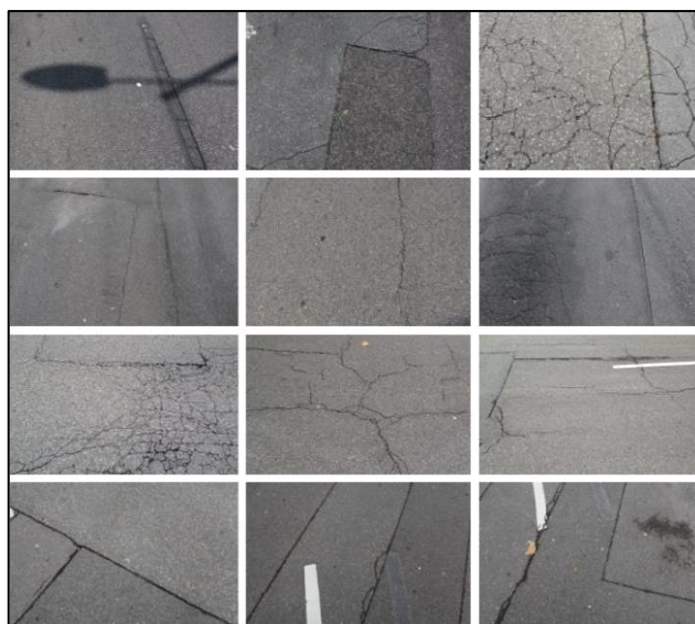
Figure 3. Some image data containing linear, block and alligator cracks
