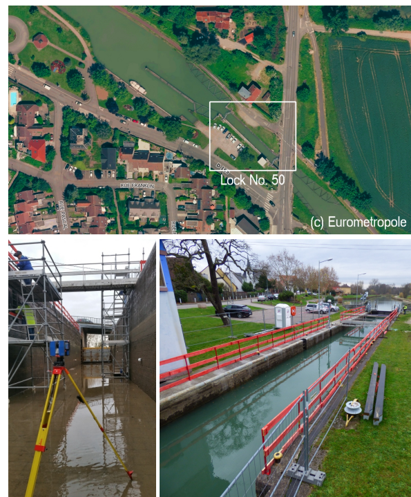
Figure 1. Top: aerial view of lock No. 50 on the Marne-Rhine canal. Bottom left: view of the lock during maintenance operations and 3D TLS surveying of the chamber; bottom right: after refilling.
