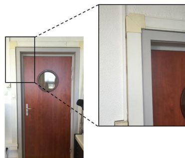
Figure 16. Example of a specific case where the cable duct surrounding door jamb would compromise acquisitions
