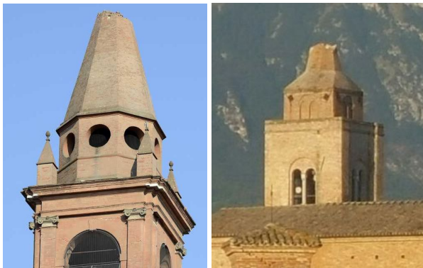
Figure 2. Damages to belfries spires in the 2012 Emilia earthquake (left) and in the 2016 Central Italy earthquake (right).
