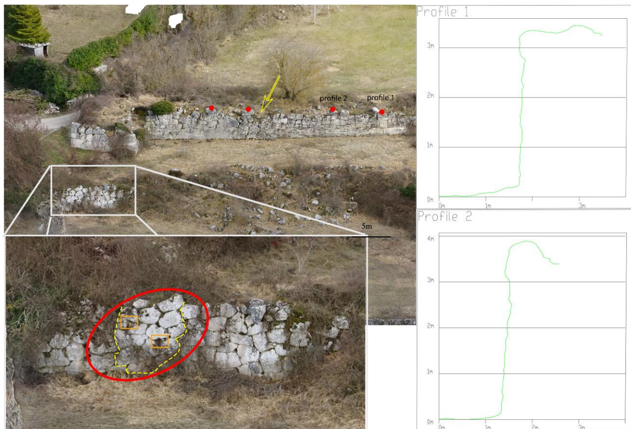
Figure 9. Degradation phenomena on the orthomosaic of the northern walls (left) and profile of the instability blocks of the walls (right).
