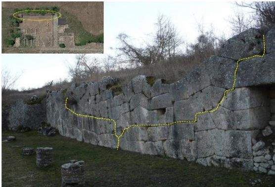
Figure 13. Megalithic wall near of the Imperial house and geotechnics function in preventing landslide: the loss of plumb line with tilting of a wall portion and production of instability phenomena (yellow dashed lines) is reported. The deformation of the wall is well observable even by common aerial application (left top frame).
