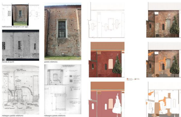
Figure 19. On the left, the process to obtain external rectified images of the Refectory using both direct measurements and laser scanner control points. On the right, the mapping process of materials and degradation pathologies of the west front of the Refectory (Laboratorio di Restauro, G. Guarisco and D. Oreni, a.y. 2016-2017)
