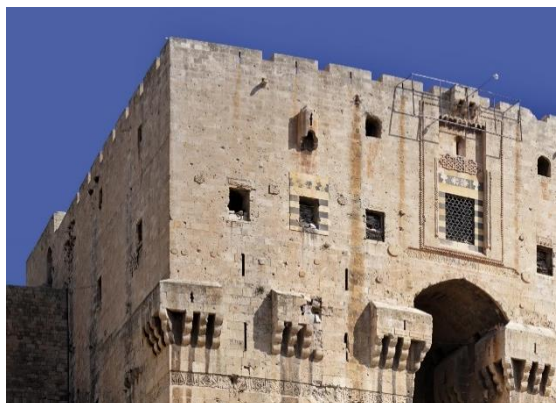
Figure 6. The entrance tower of the Citadel. The signs of the conflict are evident
