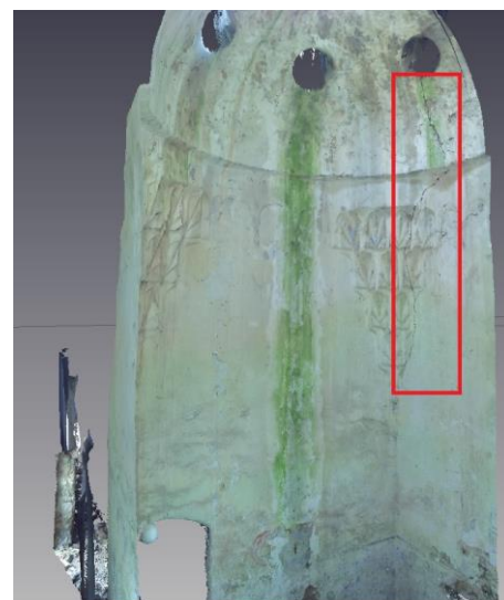
Figure 6. Wall part that contains complex surfaces and decorative motifs. The red rectangle indicates the crack position
