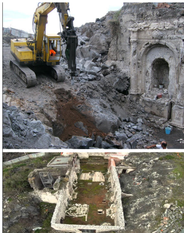
Figure 2. The excavations works at the church of Santa Maria delle Grazie in ancient Misterbianco.
