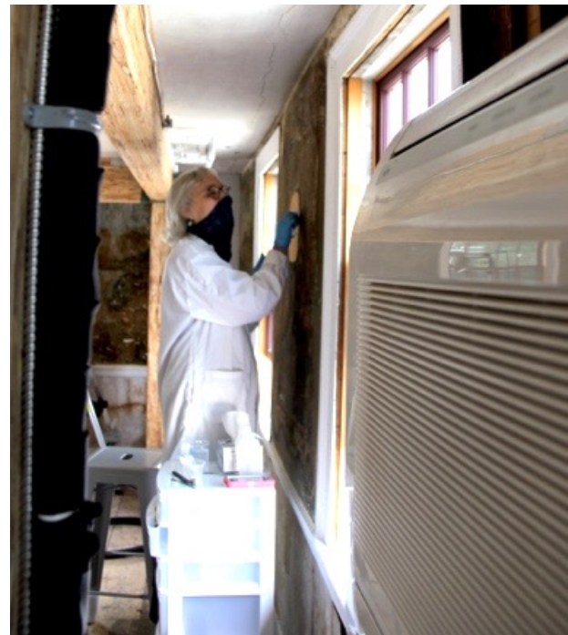
Figure 7: Conservator working next to AHS-installed environmental control unit.
