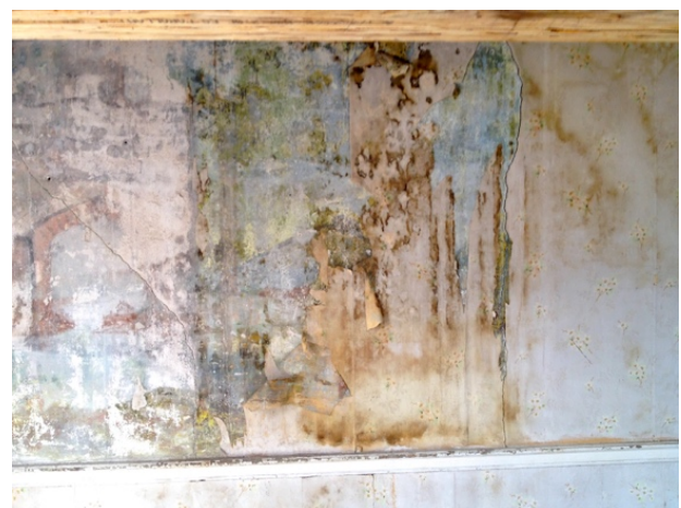
Figure 5: North wall paintings and wallpaper after roof leak. Source: Ann Shaftel
