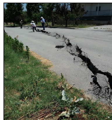
Figure 5. Ground rupture at Anargyri village due to the landslide
