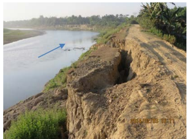
Figure 4. Embankment failure in Manu River.
