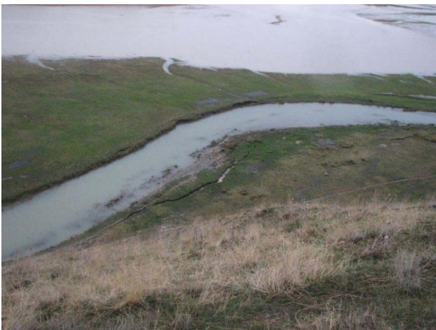
Figure 4. An example to lateral spreads from Van, Turkey, occurred after October 23 rd , 2011 earthquake (MTA, 2011).
