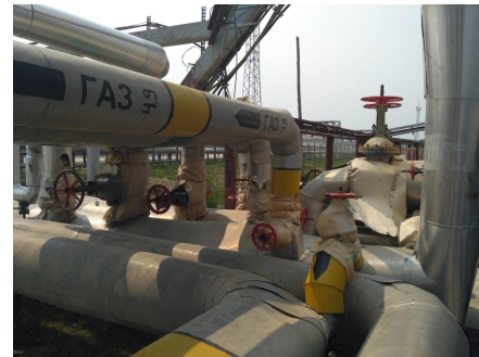
Figure 3. Digital image of a complicated area with pipelines.
