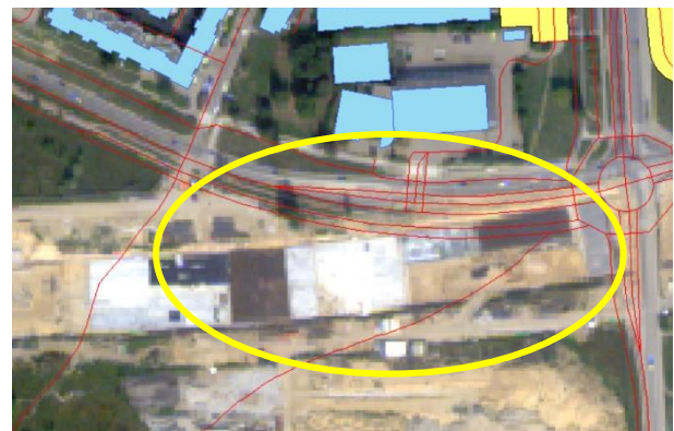
Figure 2. New road under construction. The red lines define objects in the Topographical Database.
