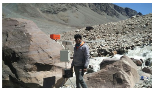
Figure 21. Installation of DWLR at downstream of Patsio glacier, H.P. (Oct. 2016). Instrument worked till April 2017, and was damaged due to heavy snowfall in 2017 winter season.
