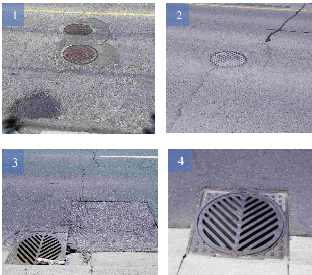
Figure 6. Captured photos from studied road surface anomalies
