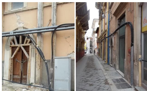
Figure 5. On the left, the temporary by-pass related to the data network (prepared by Telecom and Fastweb); on the right, the one related to the water network
