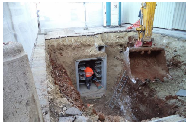
Figure 3. View of the internal part of underground tunnel set up along Corso Vittorio Emanuele II
