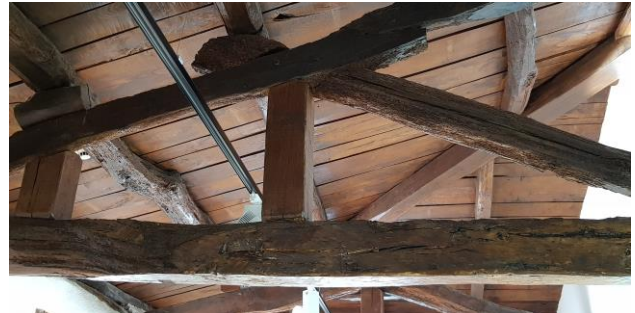
Figure 6. Detail of the wooden framework of the Álvaro Cunqueiro House Museum. Mondoñedo. Source: https://novacarta.eu .
