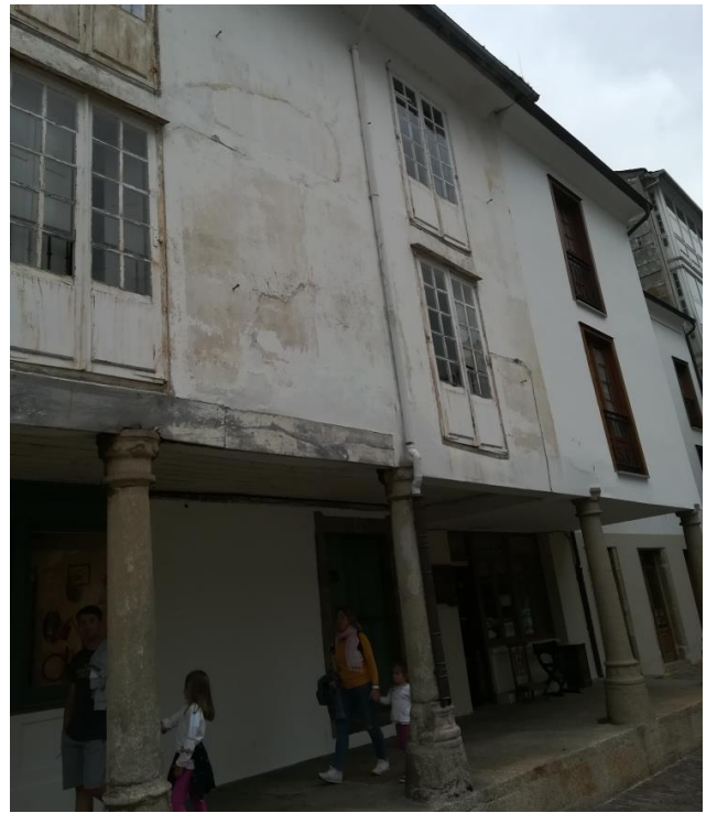
Figure 17. Half-timbered houses with large openings in the facade in Pascual Veiga Street. Source: A.F.P.
