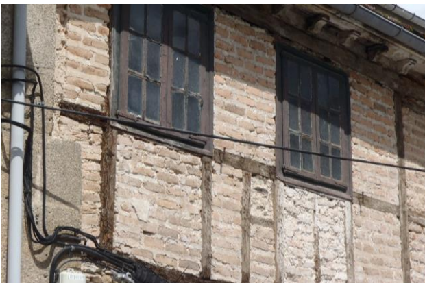
Figure 10. Detail of the half-timbered wall with brick in a house in Mondoñedo. Source: A.F.P.
