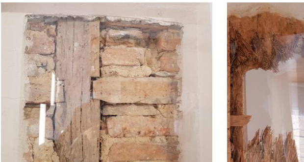
Figure 16. Details showing the half-timbered structure with the brick filling of the facade and an interior half-timbered with earth in the Álvaro Cunqueiro House Museum. The facade was made at a later time. Source: https://novacarta.eu .
