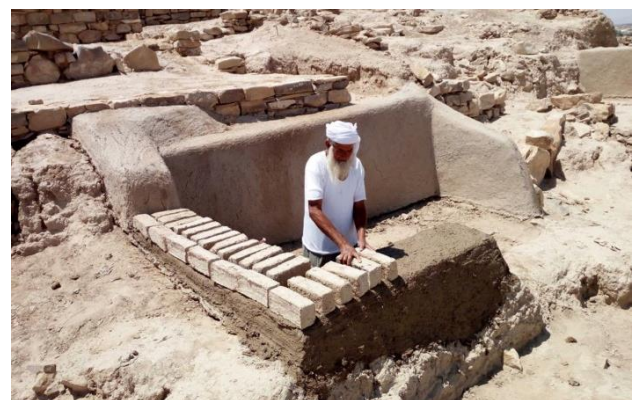
Figure 6. Mr. Massaoud Al-Khīārī rebuilding the missing part of the walls with new mudbricks made on site.
