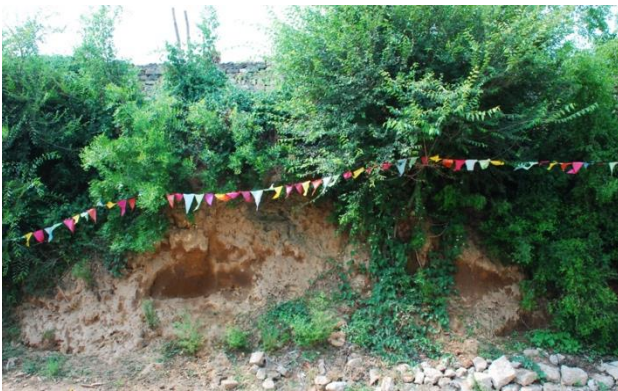
Figure 5. Present situation of peeling diseases of the south town wall.
