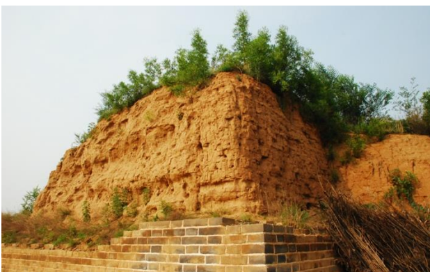
Figure 6. Present situation of weathering and collapse in the northwest corner of the town wall.
