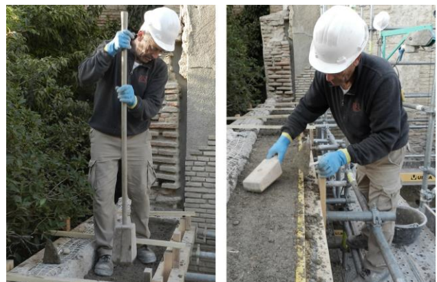
Figure 10. Manual ramming of the mass with the use of a rammer, and taping of the top surface with a hand-rammer.
