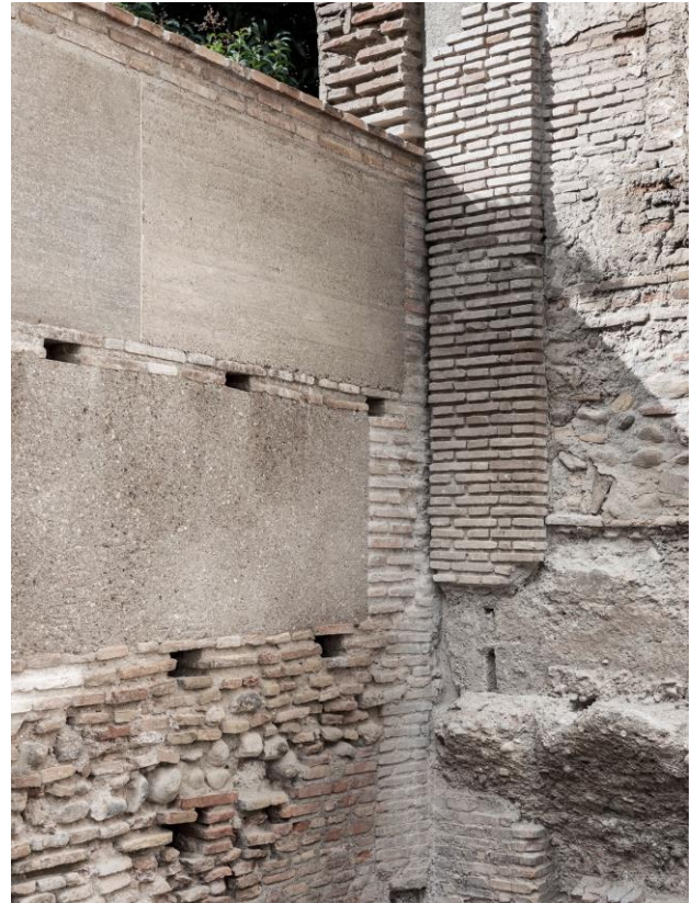
Figure 8. Final state of the rammed earth wall after the consolidation works. Photograph: Cristina García-Zarza.
