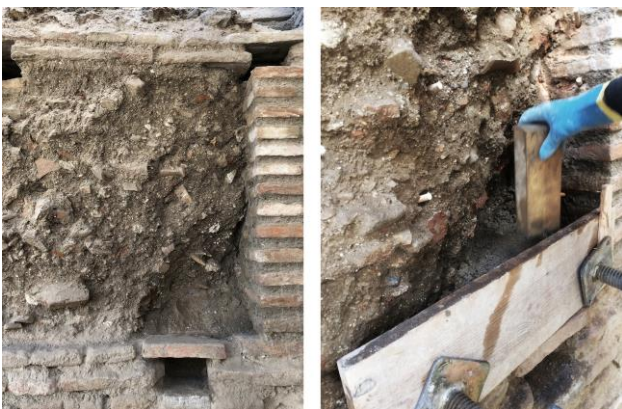
Figure 9. Detail of the previous state of the rammed earth wall with the presence of a void. Punctual formwork and ramming
