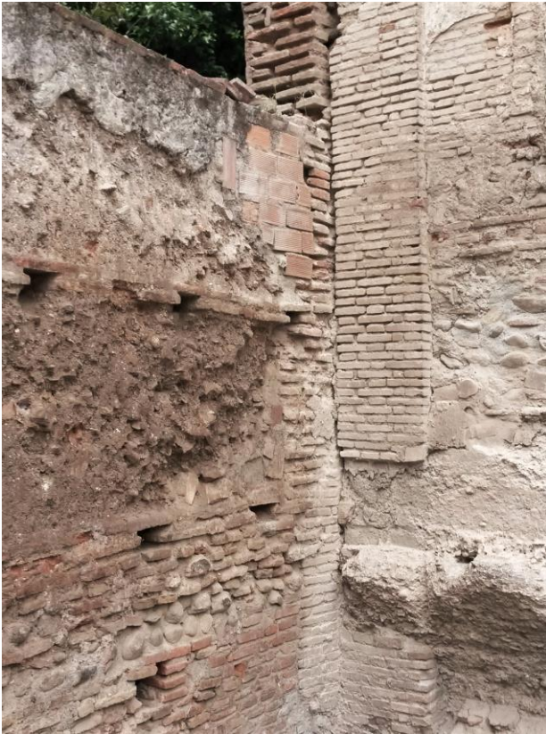
Figure 7. State of preservation of the rammed earth wall before the consolidation works.
