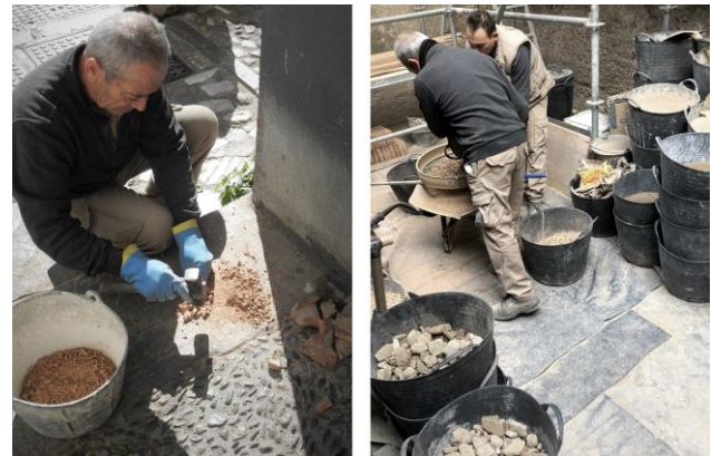
Figure 4. Chamotte preparatory works and development stage of the different masses of earth.
