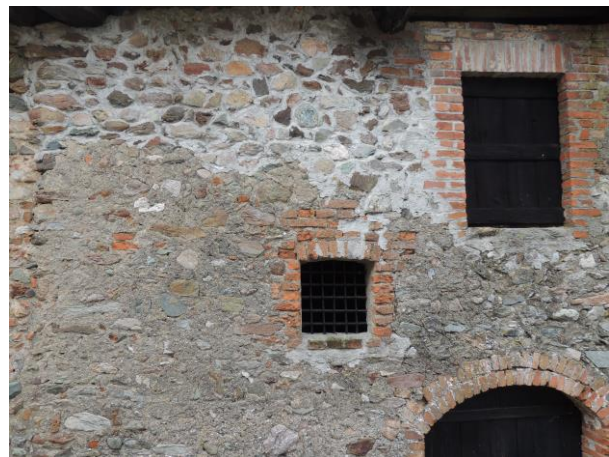
Figure 11. Building B - Reintegration of the masonry adopting inappropriate materials (credits Fabio Fratini).
