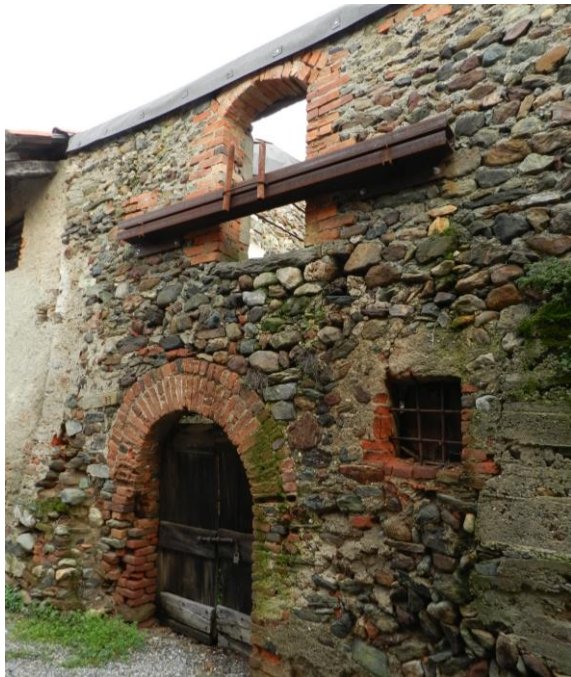
Figure 6. Building C - Temporary consolidation intervention carried out by the municipality (credits Manuela Mattone).
