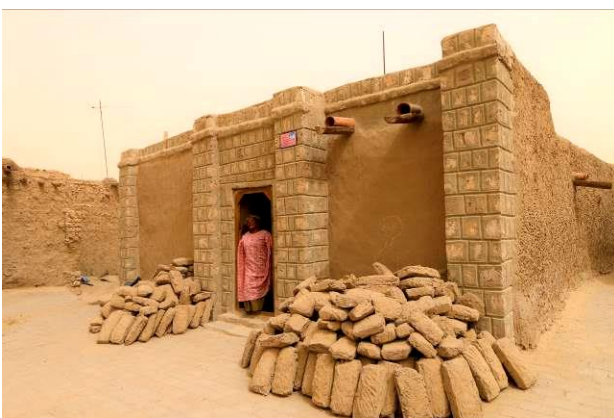
Figure 9. Restored house of widow Nana Ber, ready to carry on with additional repairs © Joffroy T. CRATERre.
