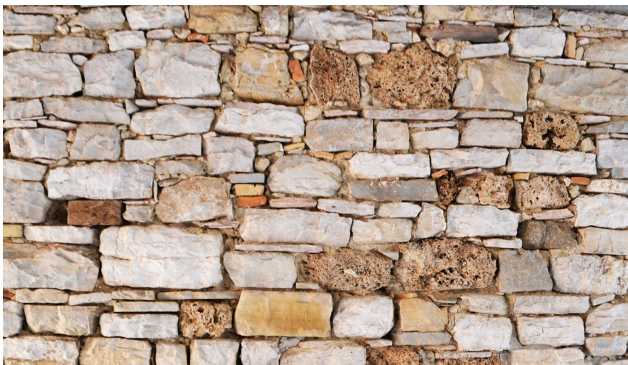
Figure 4. Frosolone (Isernia, Italy): the photo shows a masonry of limestone and cimenti (Romano, 2016).
