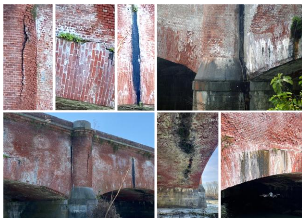
Figure 2. Examples of degradation phenomena affecting the masonry structure, including moisture infiltration and biological growth, contribute to material decay and structural weakening.
