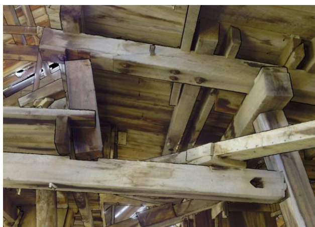
Figure 11. Failed joints showing iron fasteners
