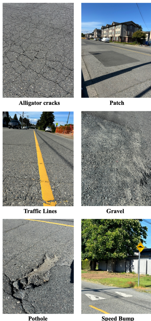
Figure 4: Types of road conditions trained for YOLOv11 for the project. These images were taken by the author at Janzen Street, Abbotsford, B.C.
