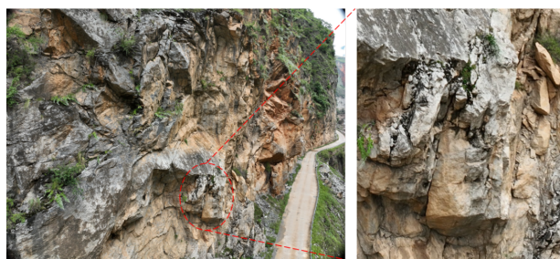
Figure 1. Representative potentially unstable rock block formed by intersecting discontinuities above the roadway.
