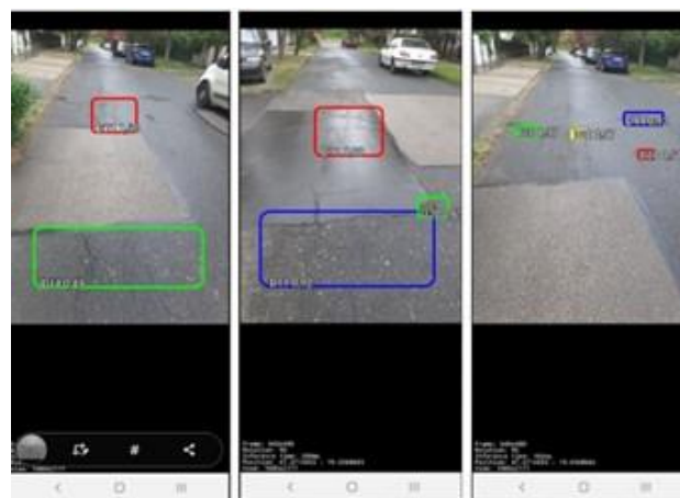
Figure 1. Road damage detected using a deep neural net (DNN) evaluation of mobile phone camera imagery
