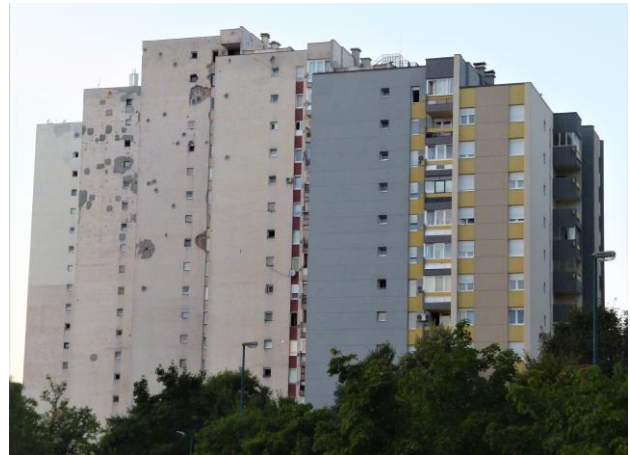
Figure 2. One of the buildings in the municipality Novi Grad that was refurbished according to standards of energy efficiency (left part of the building damaged during the war, right part refurbished).
