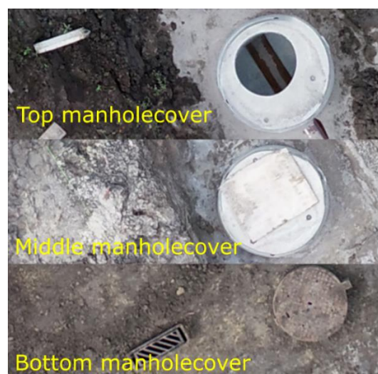
Figure 12. The three different manhole covers in detail from the construction site where the two manhole covers on top aren't finished and the one on the bottom is.
