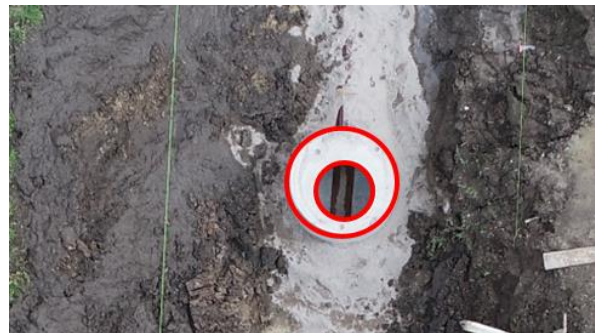
Figure 10. Manhole cover that isn't finished yet. The hole isn't centric with the pit itself.
