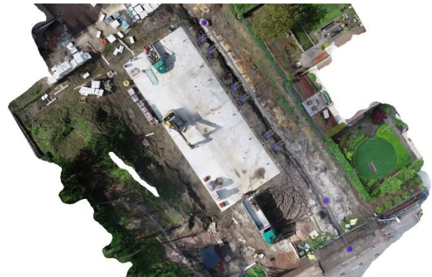
Figure 11. Detection of manhole covers out of a orthophoto compared to the as-design BIM. The two manhole covers on top of the construction site aren't finished.
