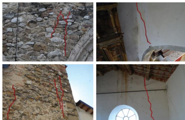
Figure 7. Detailed photographic survey on-site damages.
