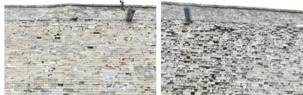
Figure 1. Bulge of the ancient wall
