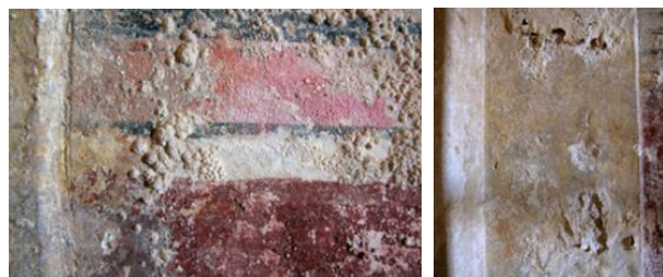
Figure 3. Efflorescence on the surface of the wall paintings at the Royal box, Herodium (Neguer & Davidoff, 2015)
