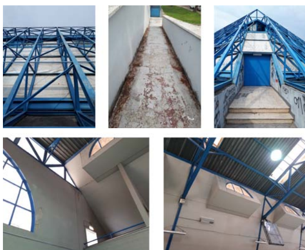
Figure 4. The state of deterioration of the good.
