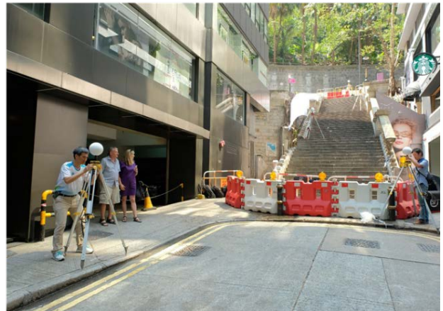
Figure 6: 3DSU conducting 3D laser scanning by terrestrial laser scanner on site after the damage.
