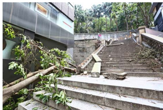
Figures 2 and 3: The Steps were seriously damaged by the fallen wall tree.
