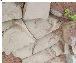
Figure.10-1 Stone stairs fracture in Fangheting
