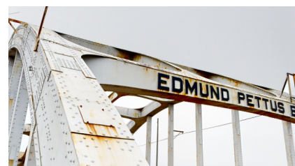
(a) Corrosion and paint maintenance needed
