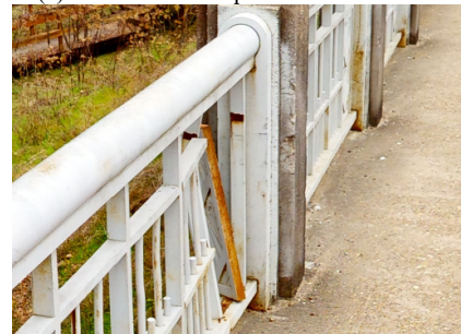
(b) Damaged railing plate and baluster
