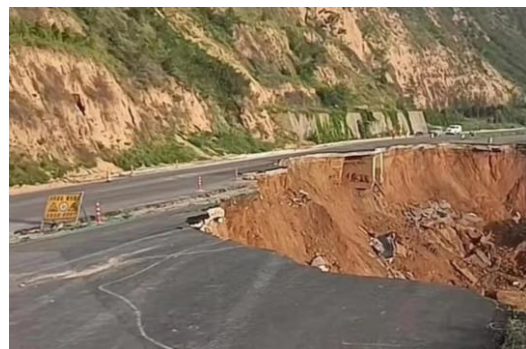
Figure 1. Collapse area of 108 national highway.
