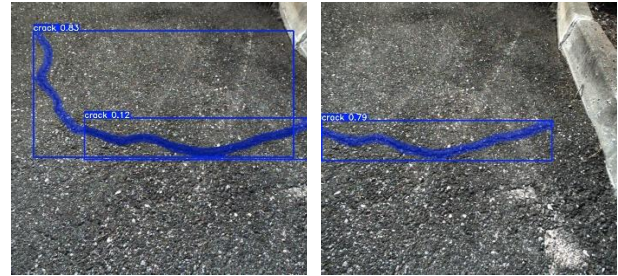
Figure 4: A pair of images with different number of segmented cracks.
