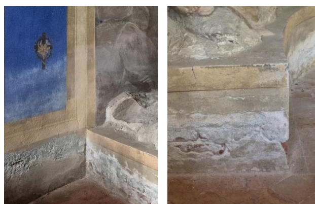
Figure 5. Detail on Chapel XVI's degradation processes
